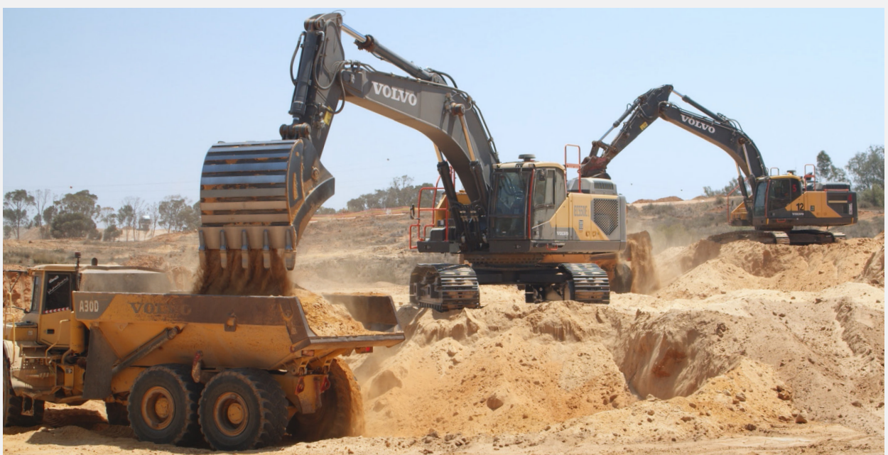
Earthworks for the new neighborhood, which involved moving 300 thousand cubic meters of earth. Photo: Guy Lumer, KKL-JNF Photo Archive
